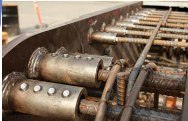
Shear-bolt couplers were welded to steel embed plates to connect longitudinal bars at the base of each wall
