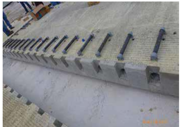
Fig. 8: Typical panel with dowel bars ready to be placed in the ducts
