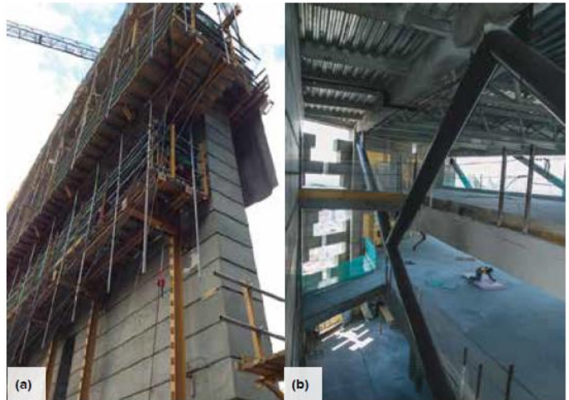
Fig. 3: Structural components of Torre Reforma: (a) shear wall formwork; and (b) atrium view of truss and perforated concrete shear wall
