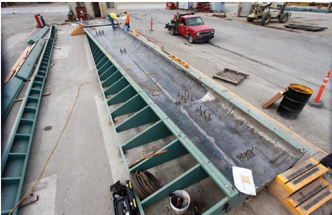
Workers are shown placing embeds in the steel form. After the reinforcing cage was installed, the top halves of the side forms were bolted in place to form the 180-degree radiused ends of the wall unit
