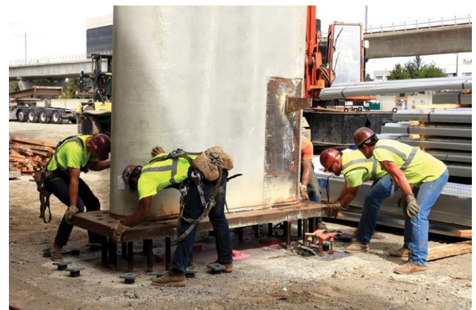
Wall units were handled using rigging inserts placed on the manually finished side, and they were anchored to foundations using cast-in-place anchor rods
