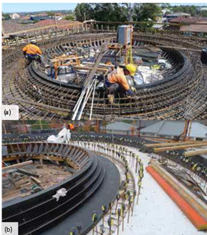
Fig.6: Ring beam construction: (a) before the first concrete placement; and (b) before the second placement (photos by Adrian Curtin, courtesy of Boral Australia)
