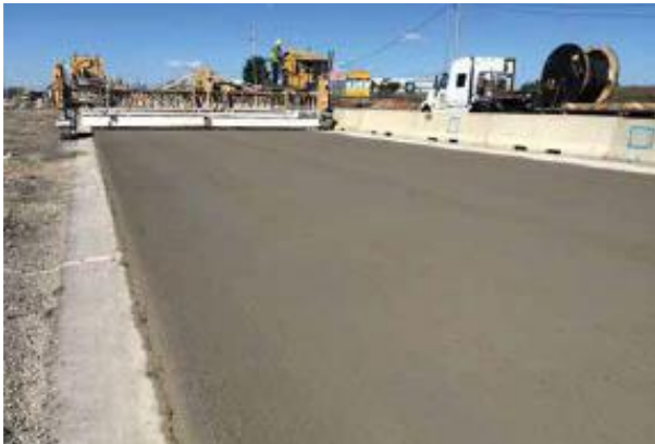
Jane Addams Memorial Tollway (I-90) Rebuilding and Widening project credits: Illinois Tollway, Owner/Engineer; Walsh Construction Company, Contractor; and Terrell Materials Corporation, Concrete Supplier
