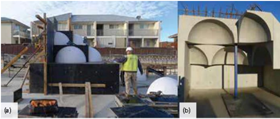
Fig. 3: A mockup was used to verify methods and materials for construction of the muqarnas: (a) formwork with molded and coated fiberglass domes; and (b) finished surface after stripping the molds (photos by Adrian Curtin, courtesy of Boral Australia)
