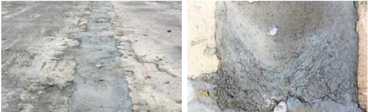
Fig. 5: Field placement after 1 day: (a) view of a UHPC connection; and (b) shrinkage cracks visible on the surface
