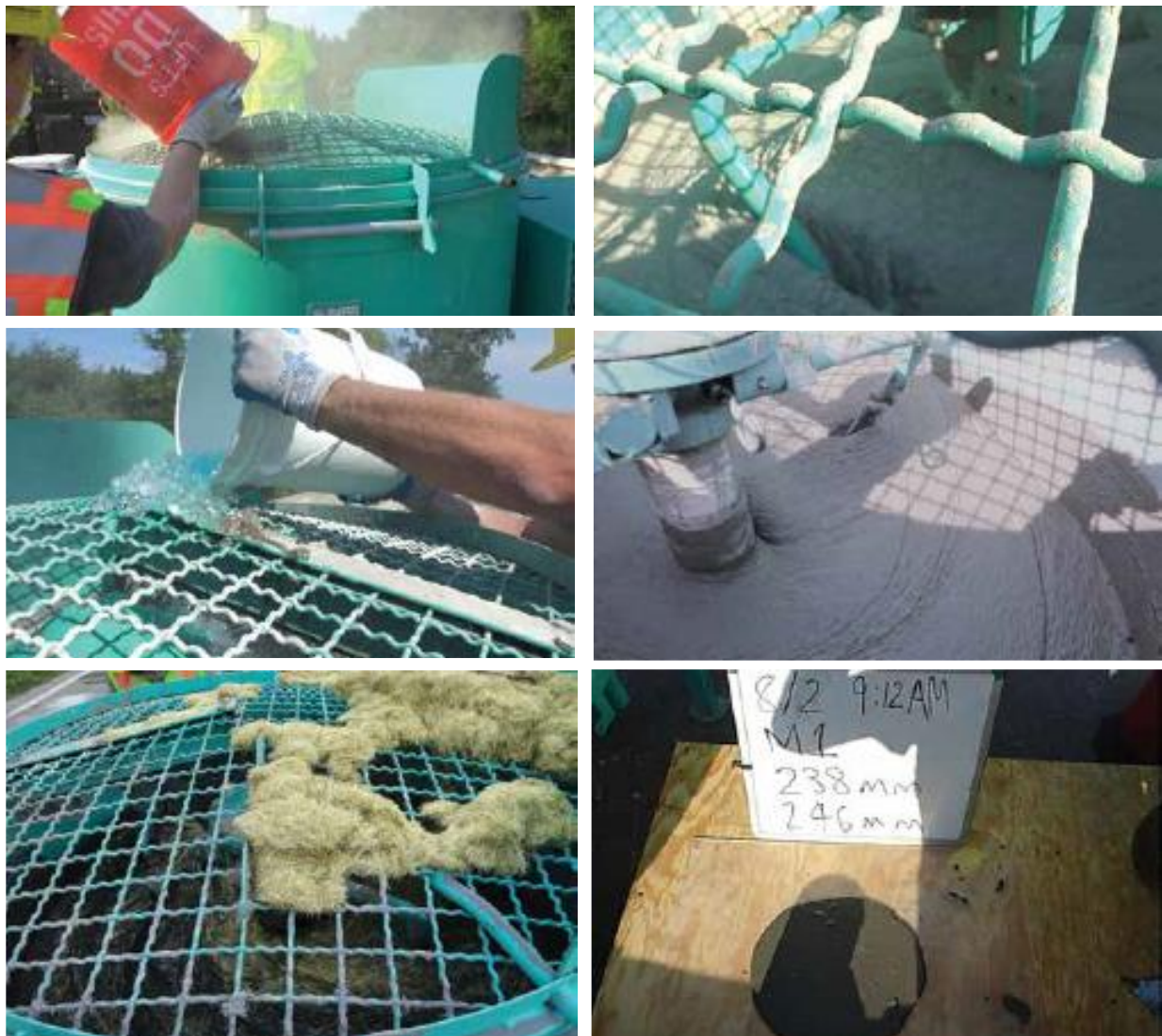
Fig. 3: Field mixing procedure and testing of UHPC mixture: (a) addition of dry ingredients; (b) dry mixing; (c) addition of water, HRWRA, and cubed ice; (d) mixture dispersion and homogenization; (e) addition of steel fibers; and (f) flow test
