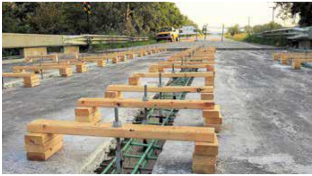
Fig. 2: Joints between reinforced concrete beams were replaced with UHPC. Dimension lumber portals and threaded rods held the bottom formwork tight against the beam flanges to prevent leakage of the UHPC
