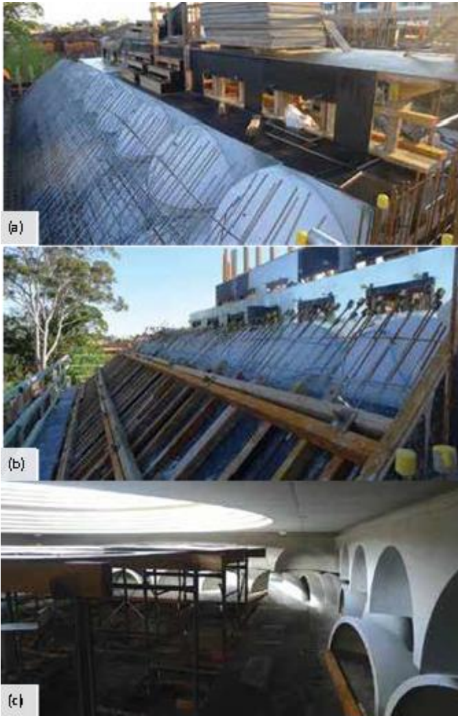
Fig. 4: Muqarnas were formed using molded fiberglass minidomes spaced 120 mm (5 in.) apart, and the flat surfaces between minidomes were formed using galvanized steel on plywood panels: (a) view of minidome forms installed on scaffolding; (b) view of exterior formwork for the sloping roof; and (c) view of minidomes during stripping operations (photos by Adrian Curtin, courtesy of Boral Australia)
