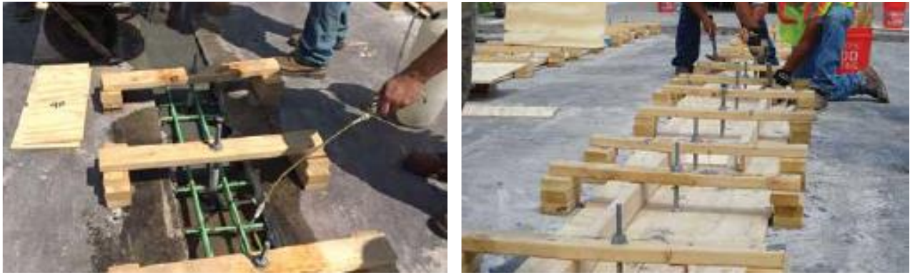
Fig. 4: Casting of UHPC into a joint between beams: (a) pre-wetting and placement; and (b) top forms installed
