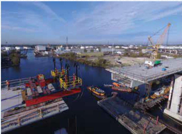
The Cline Avenue Bridge under construction. The bridge crosses The Indiana Harbor and Ship Canal
