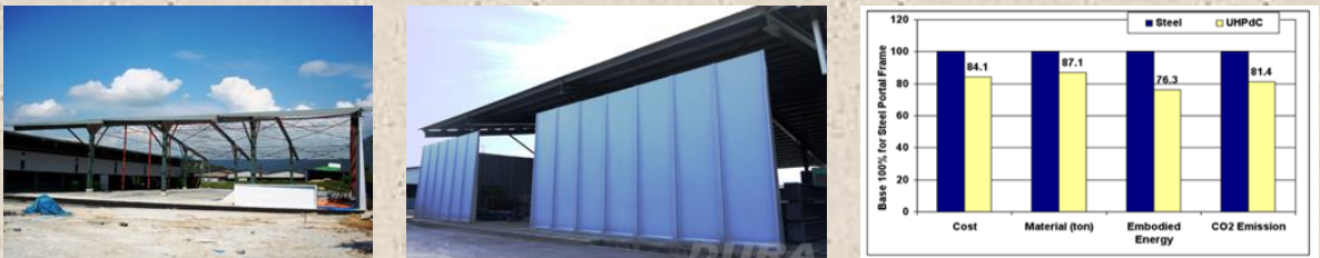
Fig. 7. Wilson Hall portal frame in Perak. (a) during construction, (b) completed structure, (c) EIC comparison with conventional steel portal frame [19].
