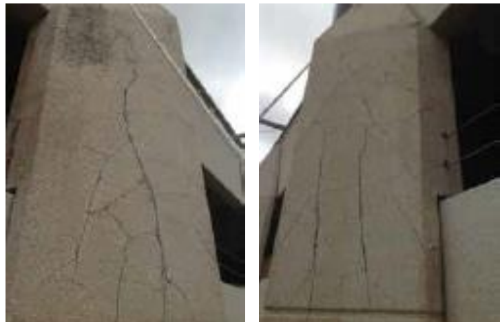
Fig. 1: Cracked load-bearing columns
