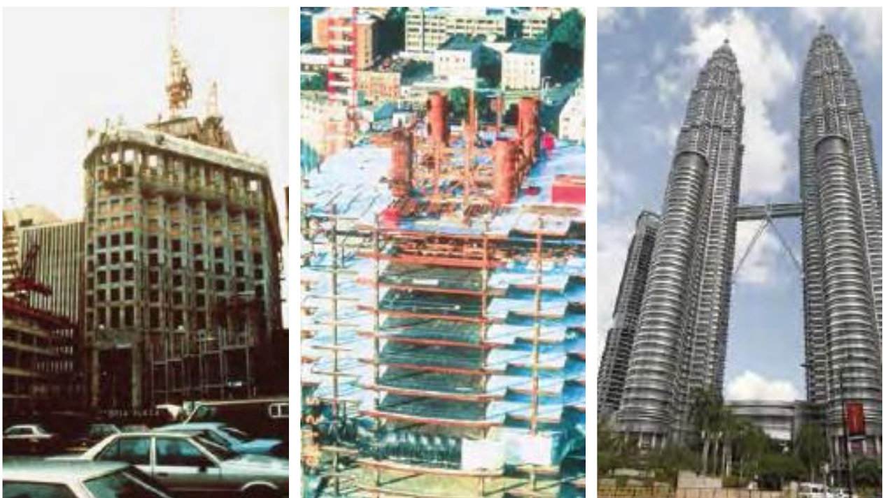
Fig. 2: High-rise building constructed with HRWRAs: (a) construction of Scotia Plaza (photo courtesy of John Bickley); (b) construction of Two Union Square (photo courtesy of Weston Hester); and (c) the Petronas Towers (photo courtesy of Morio and Wikimedia Commons)
