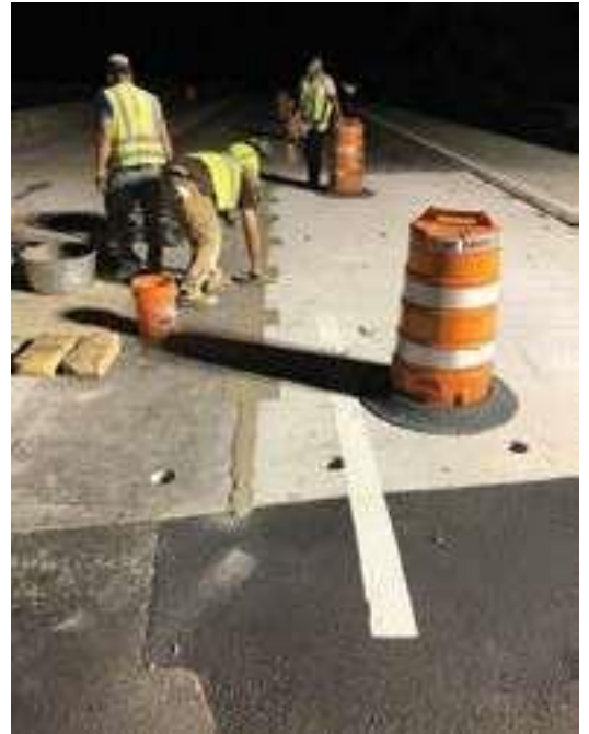
Fig. 10: Workers finish the keyway grout at the conclusion of a panel installation.
