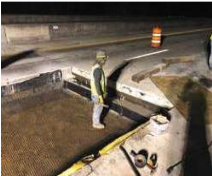
Fig. 5: The backwall seat was prepared by removing unsound concrete, repairing the seat with a high-early-strength patching material, drilling holes for the panel anchor dowels, and installing neoprene bearing pads.
