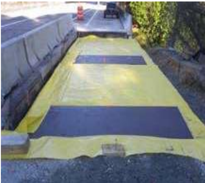
Fig. 6: Bearing plates were placed over two layers of 12 mil (0.31 mm) polyethylene sheet. The bearing plates were positioned to match the location of levelling screws in the panels.
