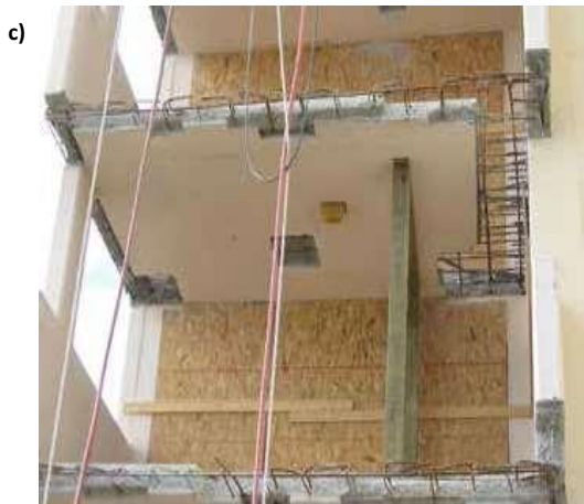
Fig. 4: Balcony repairs: (a) general construction access with visible swing stage; (b) extent of distress; and (c) one of the more severely distressed balconies requiring shoring. Note demising walls at balcony sliding glass doors.
