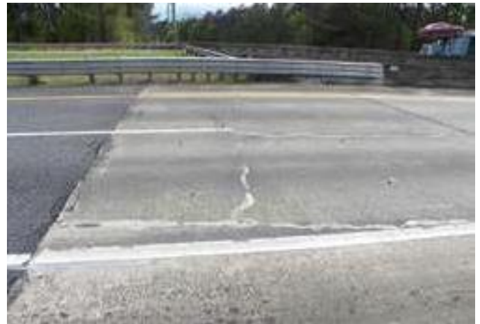
Fig. 1: The east-side bridge approach slab of westbound I-10.
