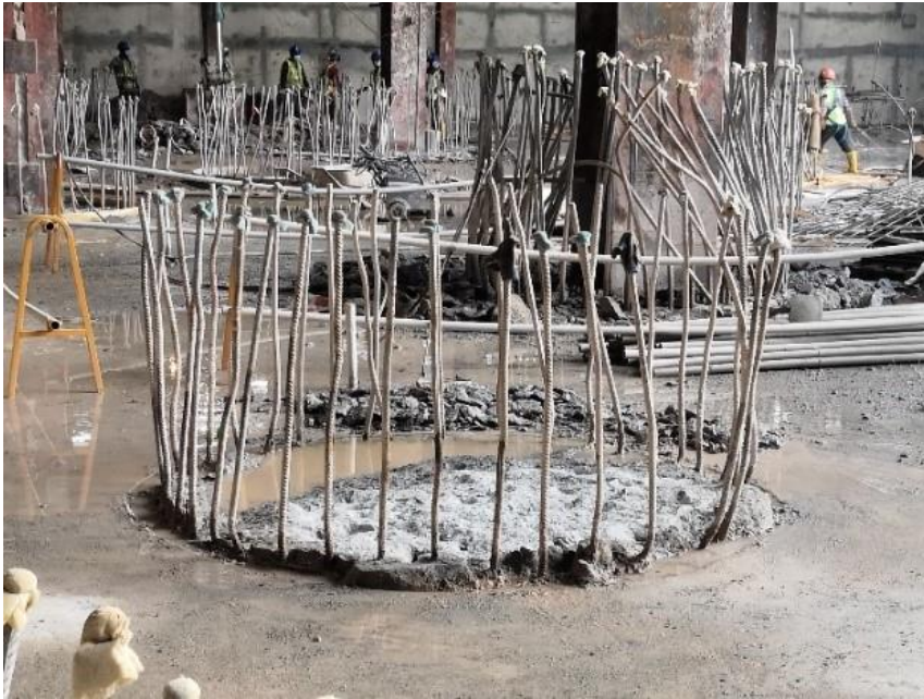
Photo 1: Uneven finishing of pile head after trimming process
