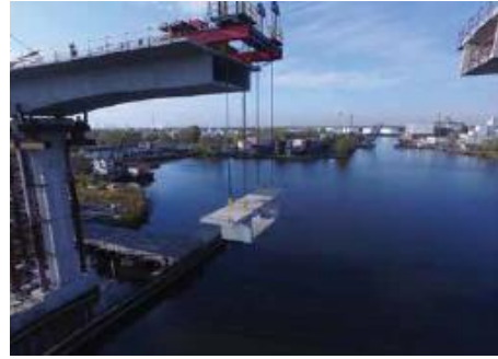
Engineered Rigging chose Enerpac strand jack technology to complete the span over the canal
