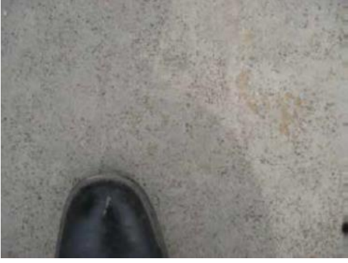
Fig. 2: Close-up look at the deck surface during inspection in June 2016, 10 years after placement
