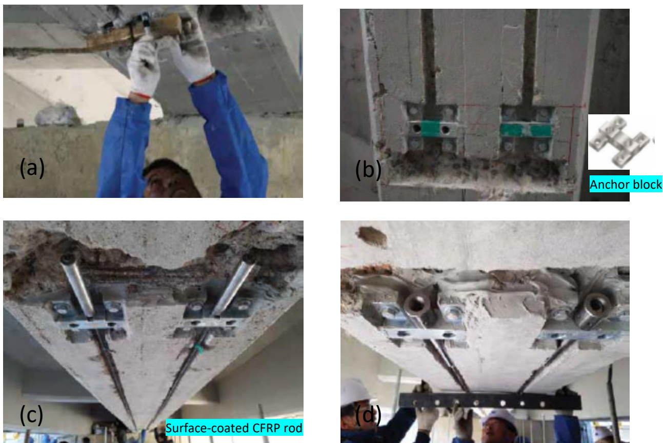
Fig. 4: Views of anchor blocks and rod anchorage sleeves: (a) a worker installs one of the four mechanical anchors used to mount an anchor block to the concrete girder; (b) installed anchor blocks; (c) anchor blocks with fixed-end anchor sleeves; and (d) anchor blocks with jacking-end anchor sleeves and fastening nuts
