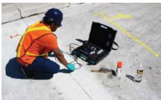
Fig. 6: A grid was applied to the surface of a repaired joint to allow locations to be correlated with UPV measurements
