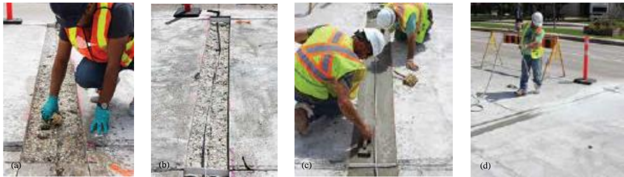
Fig. 5: After a joint had been prepared for a partial depth repair (Fig. 1 and 2): (a) the repair area was moistened; (b) a polyethylene joint former was installed at the original joint location; (c) the repair area was slightly overfilled, the mixture vibrated using a pencil vibrator, and the surface was finished with hand trowels level with the existing pavement; and (d) two coats of white-pigmented curing compound were sprayed over the patched areas as soon as bleed water evaporated from the surface
