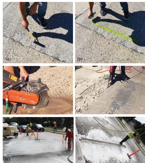
Fig. 1: Preparation of a transverse joint for partial depth repair: (a) the extent of deterioration was determined by “sounding” the concrete; (b) the boundary of the delamination was marked; (c) about 75 mm (3 in.) beyond the boundary, the pavement was sawcut to a minimum depth of 50 mm (2 in.); (d) the deteriorated concrete was removed with a demolition hammer; (e) the repair area was shot blasted to remove loose particles; and (f) remaining residue was removed using a compressed air wand.
