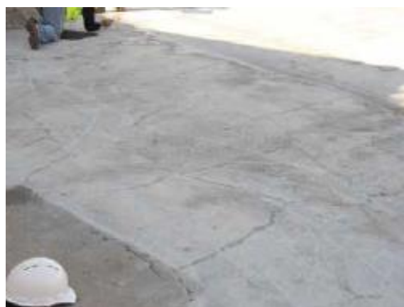
Fig. 4: Typical restrained shrinkage cracking observed in the Glen Elder Dam spillway repair areas (based on Reference 1). This cracking prompted a review and adjustment of the concrete mixture used for subsequent repairs
