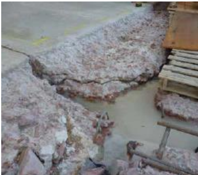
Fig. 6: Delamination at a depth of 6 to 10 in. (150 to 250 mm) of the Fort Randall Dam spillway visible after initial removal (U.S. Army Corps of Engineers, June 16, 2014)
