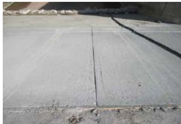
Fig. 7: A concrete overlay shown at 29 days after placement exhibits no shrinkage cracking. This overlay comprised a 25 x 25 ft (7.6 x 7.6 m) monolithic placement (U.S. Army Corps of Engineers, Oct. 11, 2013)
