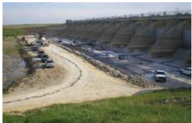
Fig. 1: View of repair work for the inlet apron slabs on the upstream side of Glen Elder Dam spillway. There is no water in contact with the spillway unless the reservoir is in the flood pool
