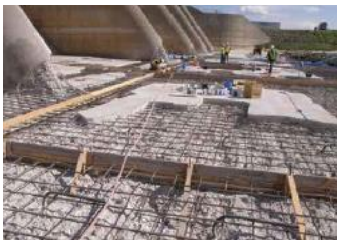
Fig. 2: Inlet slabs and spillway structure prior to placement of overlay concrete. The hooked bars that extend over the top mat are foundation anchors (No. 11 bars grouted into the underlying rock)
