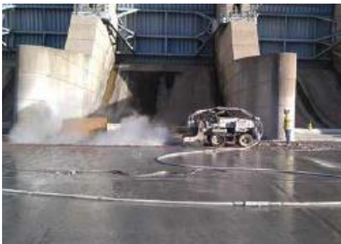
Fig. 5: Hydrodemolition of the upper expansion joint at the Fort Randall Dam spillway (U.S. Army Corps of Engineers, Oct. 1, 2013)
