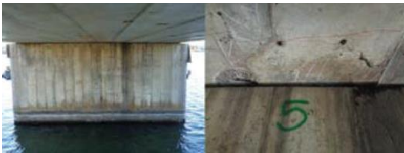
Fig. 6: The underside of the LaSalle Causeway bridge deck exhibited visible damage only near the central pier
