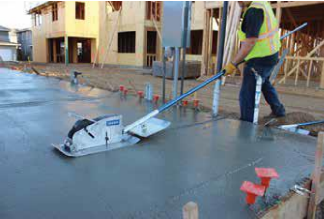
Fig. 5: This manually operated tool is used to embed a polymer tape into fresh concrete. The tape creates a stress concentration in the hardened concrete, typically resulting in a relatively straight crack that opens as the concrete shrinks (photo courtesy of Aaron Hilbert LLC)
