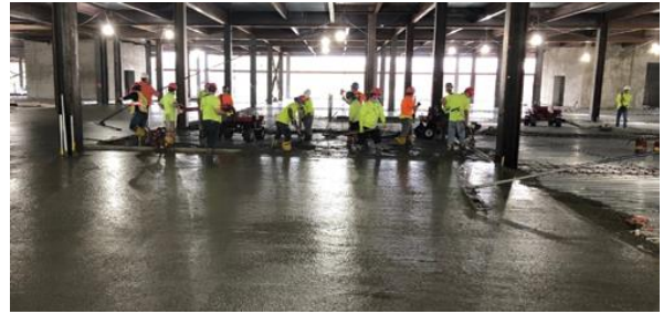
Fig. 2: A concrete placement on an elevated floor in a hospital in Ridgewood, NJ, USA. The concrete slab on a metal deck was reinforced using only synthetic macro fiber reinforcement
