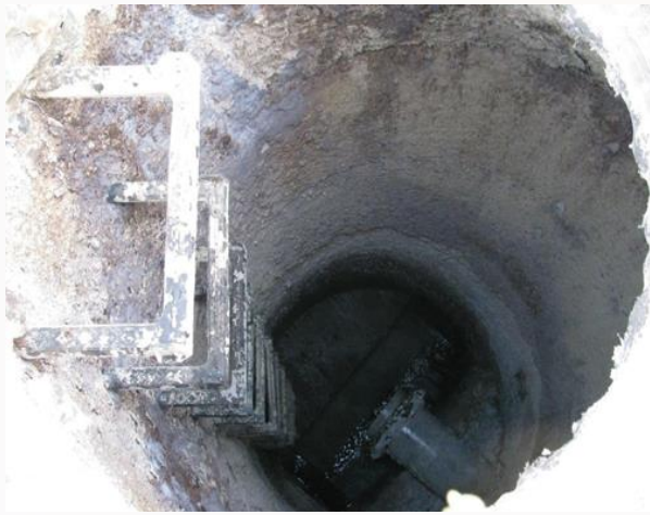
Fig. 2: Calcium sulfate (gypsum) forms a whitish foamy mass on concrete
