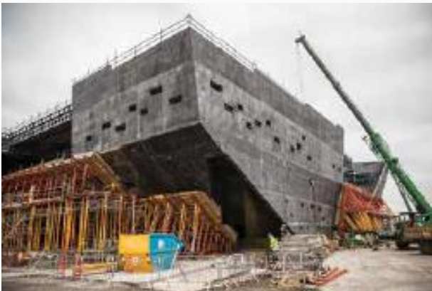
Fig. 8: Façade walls remained propped until the internal floor plates, beams, and slabs were fully tied into the structure and the concrete had reached design strength
