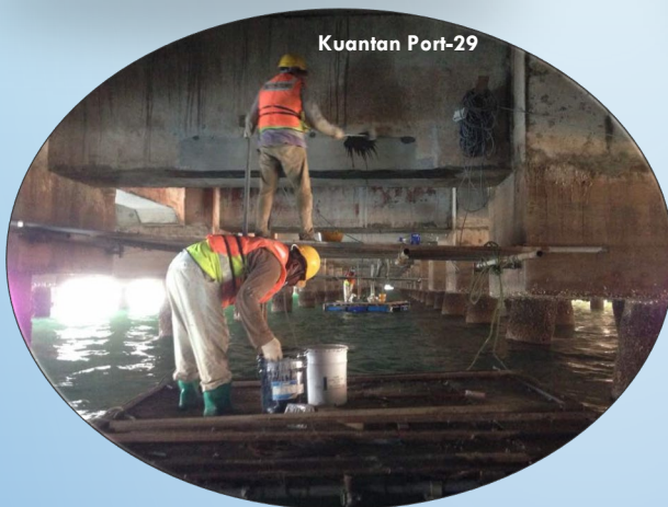
Splash water on the surface for the first 24 hours of curing to avoid surface cracks from plastic shrinkage.
