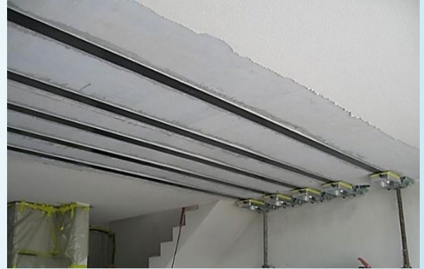
Fig. 4. Real life picture of externally prestressed CFRP bonded strengthened building, Ebikon, Switzerland (CH) [6]
