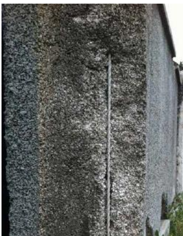
Fig. 3: An example of a square twisted reinforcing bar in the pervious concrete wall at the Rosehill Cemetery, Chicago, IL. Spalling damage can be seen at the interface between the pervious wall beyond and top of the bearing surface of the foundation. The foundation is composed of similar porous concrete covered with a mortar coating approximately 1/8 in. (3 mm) thick
