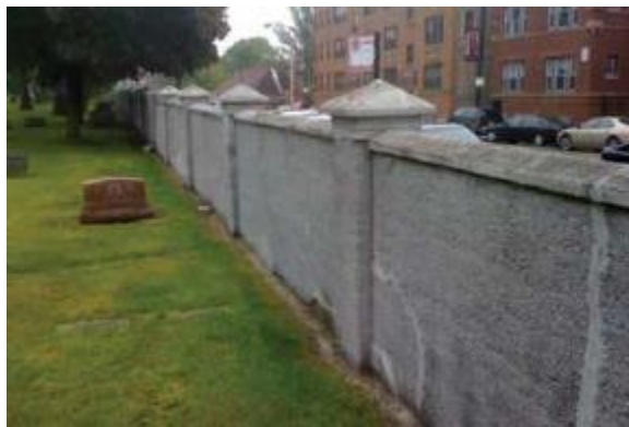
Fig. 1: Overall view of the Rosehill Cemetery, Chicago, IL, perimeter wall, which comprises porous concrete. The coping (top cap) is similar porous concrete but is covered with a mortar coating and exhibits occasional damage due to freezing-and-thawing. The wall exhibits corrosion-related distress, particularly near the base, where the pervious concrete is supported by a foundation made of similar porous concrete covered with a mortar coating approximately 1/8 in. (3 mm) thick
