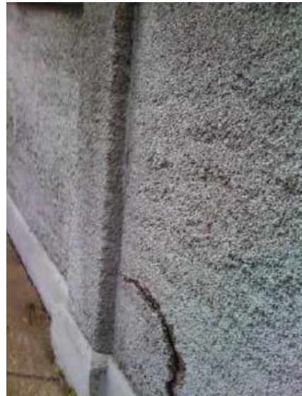
Fig. 6: The frequency and severity of distress is predominately greater at the base of the pervious wall, where the pervious concrete bears on the closed surface of the mortar-covered concrete foundation
