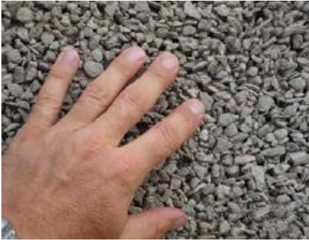
Fig. 4: Texture of exterior face of pervious wall. The mixture contains 5/8 in. (15.9 mm) crushed aggregate and a small amount of sand. Form board impressions are occasionally evident, but very few lift lines are visible, suggesting thorough mixing, efficient placement, and methodical consolidation (probably by tamping)
