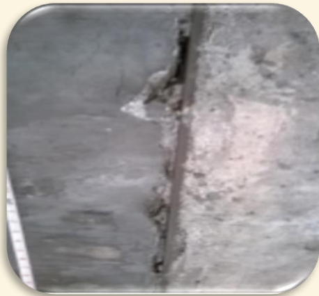
Figure 1. Damage at joint.
