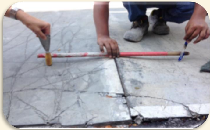
Figure 2. Curling at slab edge.
