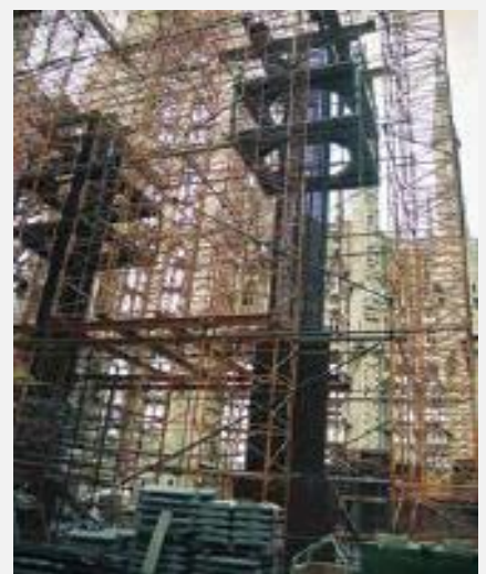
Fig. 5: Construction of the interior columns was completed inside the existing façades between 1991 and 2003 (© Fundació Junta Constructora del Temple de la Sagrada Família)
