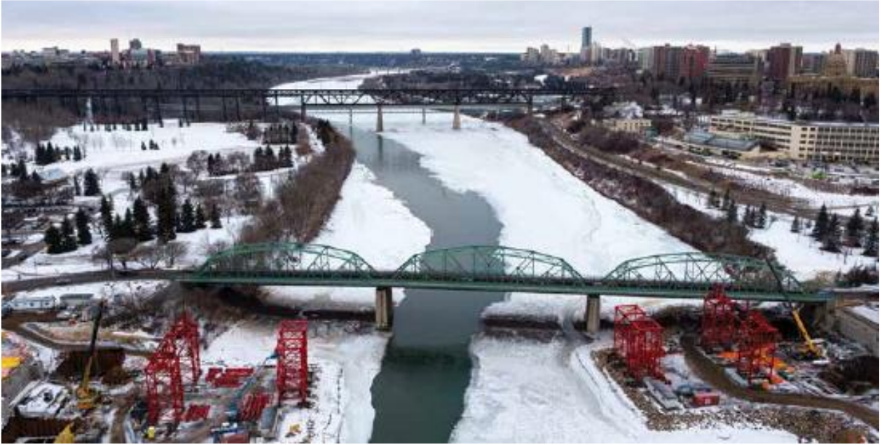
Skymatics used its drone to capture images of the new Walterdale Bridge project in Edmonton, AB, Canada
