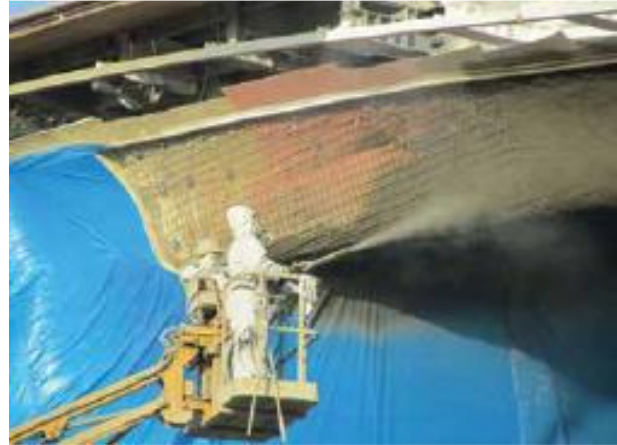
Fig. 10: Shotcreting process. In the lower section of the photo, the finished shotcrete wall is covered with plastic sheets to protect it against contamination by mortar overspray and provide curing to limit drying shrinkage
