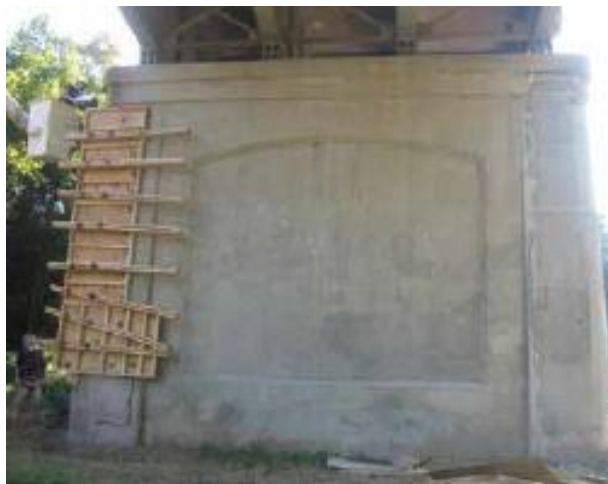
Fig. 8: Final stage of the SCC repair on one of the piers of Route 340 bridge. On the right hand side of the pier is the completed repair
