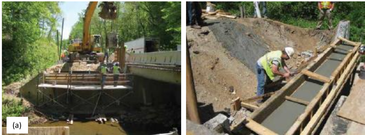
Fig. 6: Backwall repair on Route 699 bridge: (a) SCC was placed using a bucket; and (b) in the background, a sample of the SCC exhibited good stability, as the aggregate and paste in the mixture reached the bottom of the slope simultaneously
