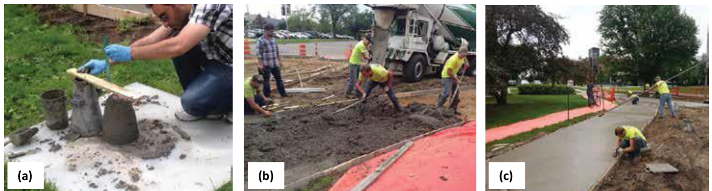
Fig. 5: Field trial operations with geopolymer concrete: (a) slump test; (b) spreading; and (c) finishing
