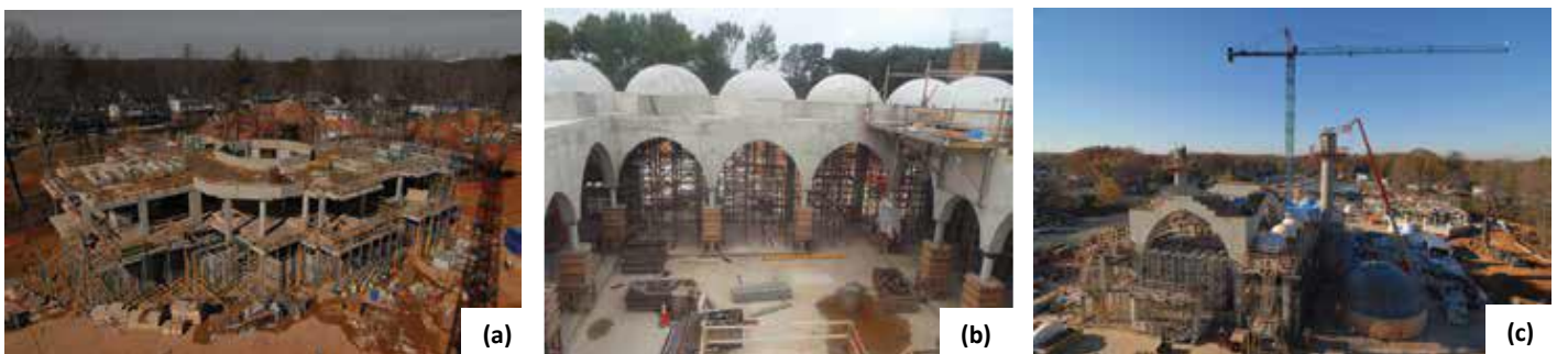
Fig. 6: Multiple shoring and decking solutions were used for construction of the project: (a) elevated floors in the Turkish bath were formed using PERI MULTIPROP shoring, formwork girders, SKYDECK panel slab formwork supplied by PERI Formwork Systems, Inc., along with HICO beams provided by Form Service, Inc. (photo courtesy of Mostafa Fahimi, EyeConstruction, Inc.); (b) formwork for the small domes surrounding the mosque courtyard were supported on Harsco 20K steel shoring (photo courtesy of Facchina Construction Company, Inc.); and (c) support for the main dome arch formwork and the work platform below the main dome formwork were provided by Harsco GASS aluminum shoring and joists (photo courtesy of Mostafa Fahimi, EyeConstruction, Inc.)
