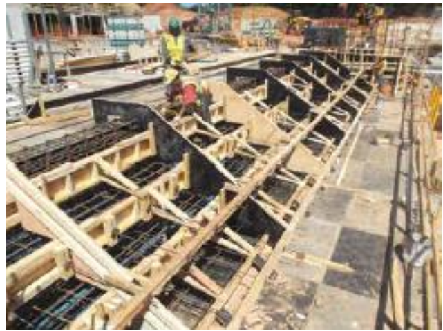
Fig. 12: Seating areas in the Turkish bath were formed using dimension lumber and plywood sheathing (photo courtesy of Facchina Construction Company, Inc.)
