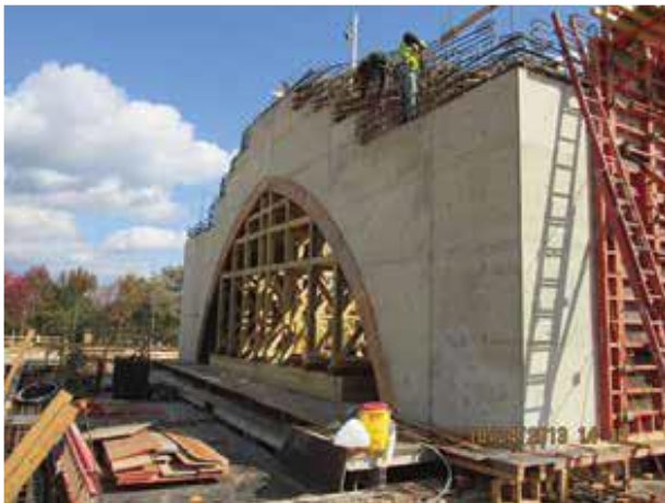
Fig. 8: The mosque structure included a platform for the main dome supported on four arched beams. The arched beams were formed using a combination of shored structural laminated timber to form the arch and PERI TRIO panel formwork to form the sides (photos courtesy of Facchina Construction Company, Inc.)
