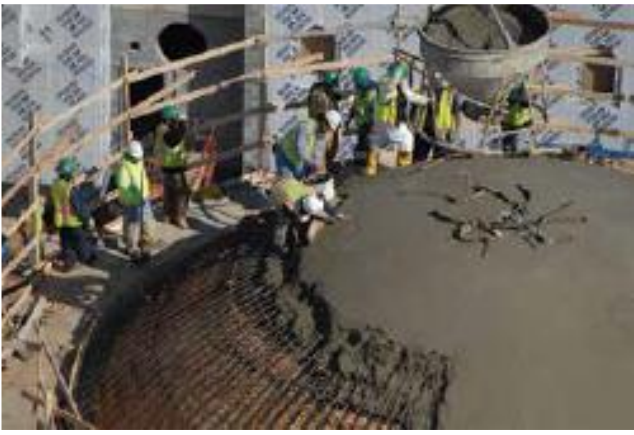
Fig. 10: Workers place concrete on the main dome of the mosque. The final depth and shape of the dome were achieved using a depth gauge and a curved screed (photo courtesy of Mostafa Fahimi, EyeConstruction, Inc.)
