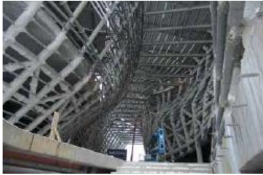
Fig. 6: The concrete and steel structure of the museum's entry hall defined the basic form of the undulating interior walls
