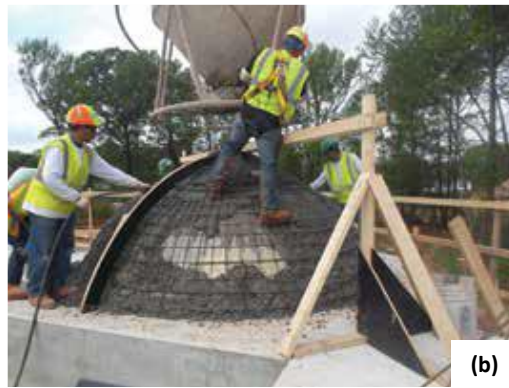
Fig. 7: The multiple small domes on the mosque and Turkish bath were formed using EPS foam blocks cut to the required radius: (a) after the dome forms were set on a shoring and decking platform, plastic sheets and nylon straps were taped over the casting surface (to ease stripping), and a pre-assembled reinforcing cage was placed; and (b) a 2 to 5 in. (50 to 125 mm) slump concrete mixture was applied using a template and depth gauge to set the thickness (photos courtesy of Facchina Construction Company, Inc.)
