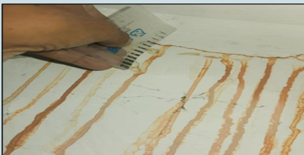
Photo 3: Cracks at soffit of slab with cracks size of 0.6mm wide with rust stain from corroded rebar.
