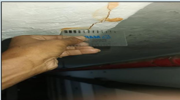
Photo 2: Cracks at soffit of slab with cracks size of 1.2mm wide
