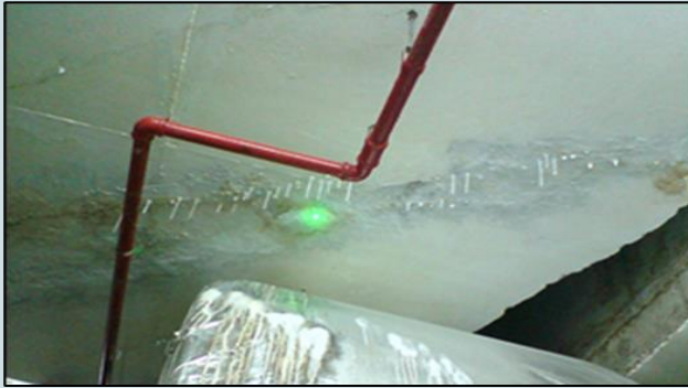
Photo 1: Cracks at soffit of slab with stalagmite formation due to leaks
