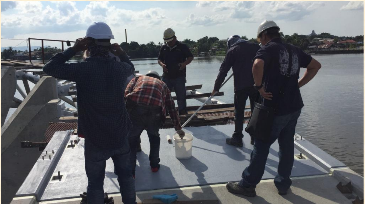
Application of Mapefloor Finish 57 to provide a good abrasion- and chemical- resistant finish
