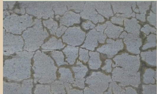
Figure 2. Pattern cracking due to alkali silica reaction [12]
