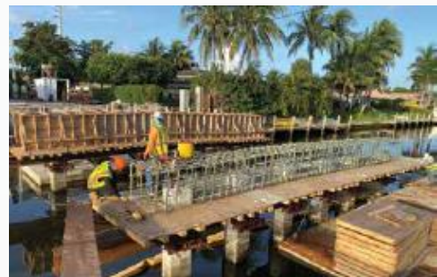
Fig. 4: A coastal bridge under construction. The piers and bent cap were reinforced with FRP reinforcing bars supplied in both straight and pre-bent forms
