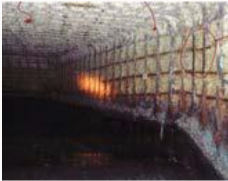
Fig. 7: Sewer tunnel with exposed second mat of steel reinforcement. Top concrete and the first mat of steel reinforcement were reportedly lost to the existing surface (from Reference 7)
