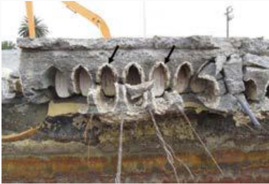
Fig. 2: Fractured concrete roof panel. BSA-caused deterioration manifested as paste color lightening and weakening along the cell perimeter (arrows) as well as corroded and broken prestressing strands
