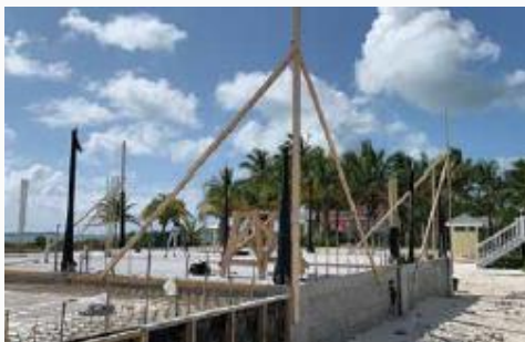
Fig. 3: A coastal residence under construction. The concrete slabs, concrete columns, and masonry walls included FRP reinforcement
