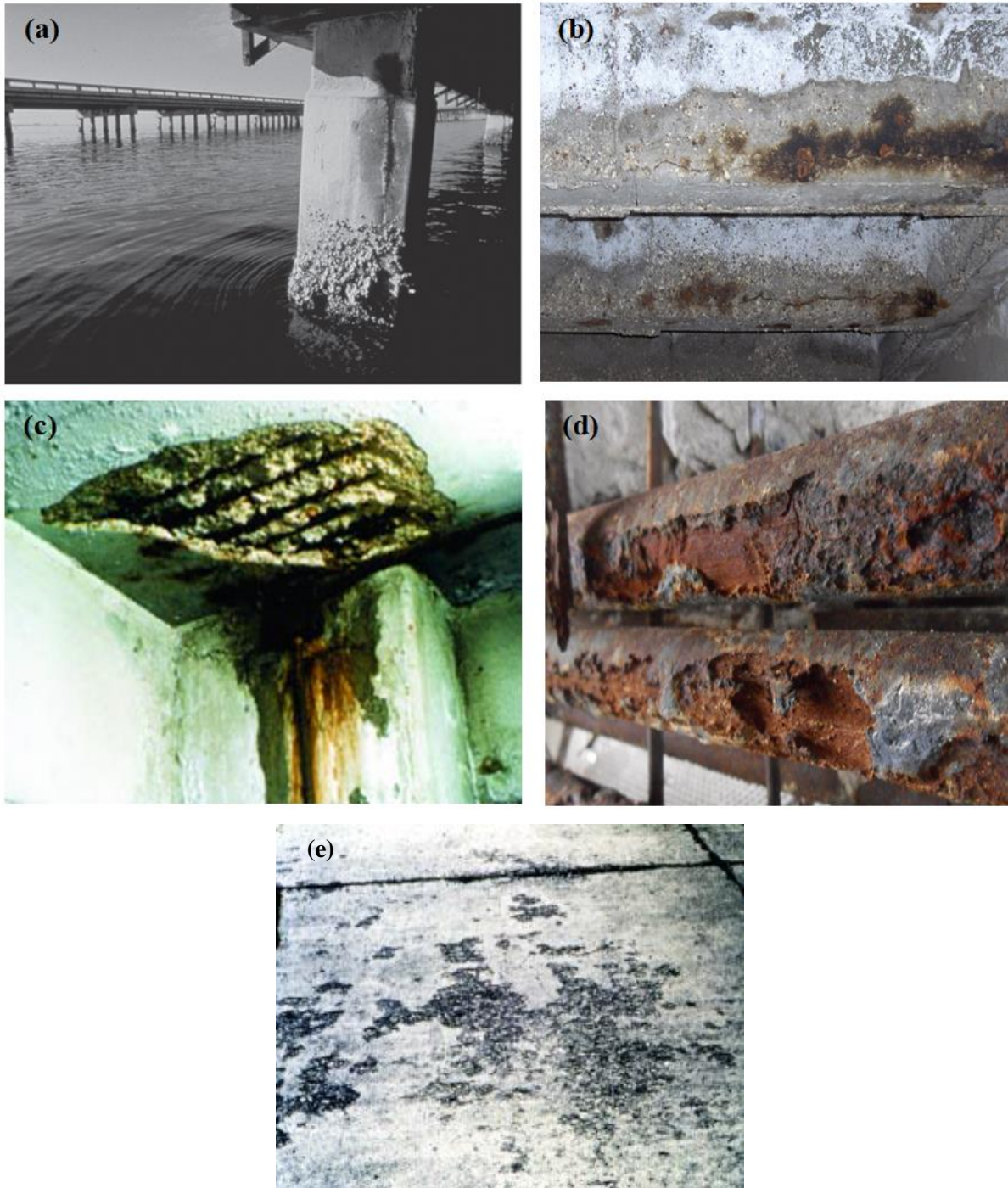
Figure 1: Example cases of primary mechanism of the deterioration by (a) cavitations, (b) sulphate attack, (c) reinforcement, (d) carbonation and (e) freezing and thawing
