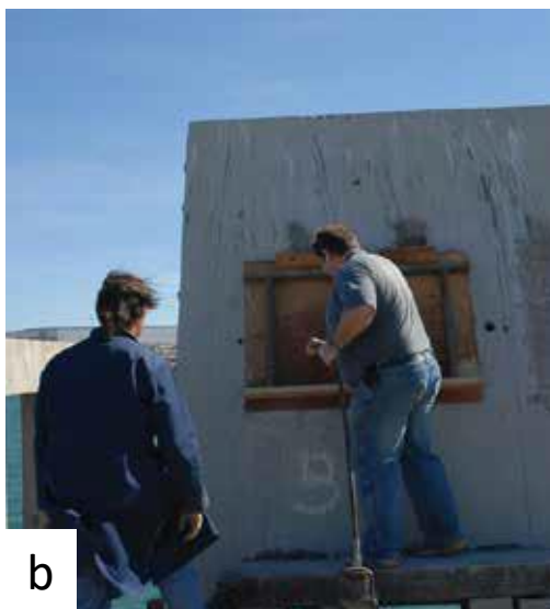
Fig. 6: Repair areas selected for field experiments at the U.S. Navy facility in Port Hueneme, CA, USA: (a) horizontal, on the pier, 73.5 x 19.5 in. (1840 x 490 mm) and 3 in. (75 mm) deep; and (b) vertical, on an existing slab installed upright next to the selected pier, 48 x 36 in. (1200 x 900 mm) and 3.5 in. (88 mm) deep.
