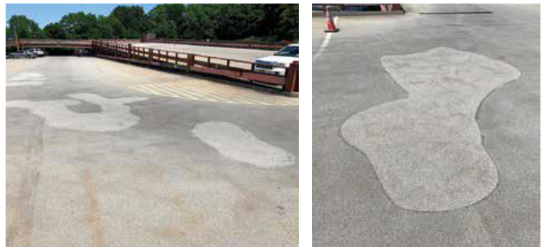
Fig. 7: A parking garage deck in Utica, NY, USA, repaired with the rubber-modified repair material, after 4 years in service
